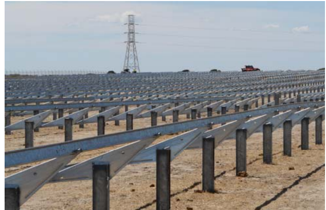
The tables have been installed at Greenough River Solar Farm. A high voltage transmission line runs past the site.
