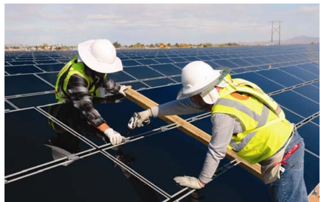
PV arrays like this will be installed at Greenough River Solar Farm.
